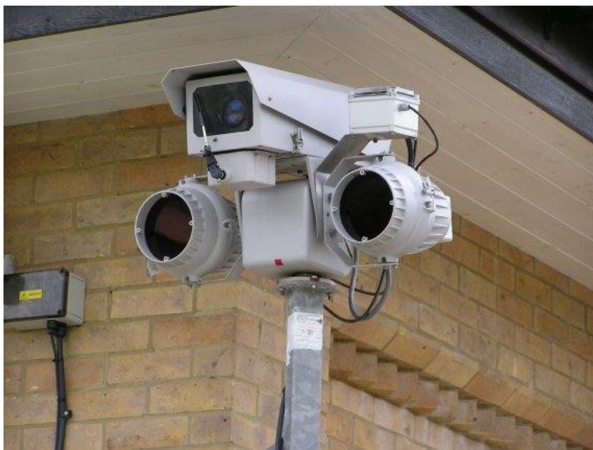
Figure 4.3: Outdoor CCTV Camera in University of Cambridge
